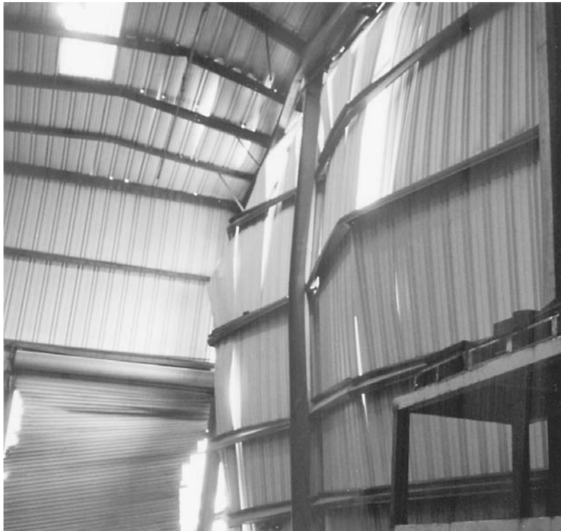
FIGURE 10.17 This building in Southern California partly failed under wind loading. Note buckling of endwall girts and roof purlins and failure of overhead door. (Photo: J.R. Miller & Associates.)
